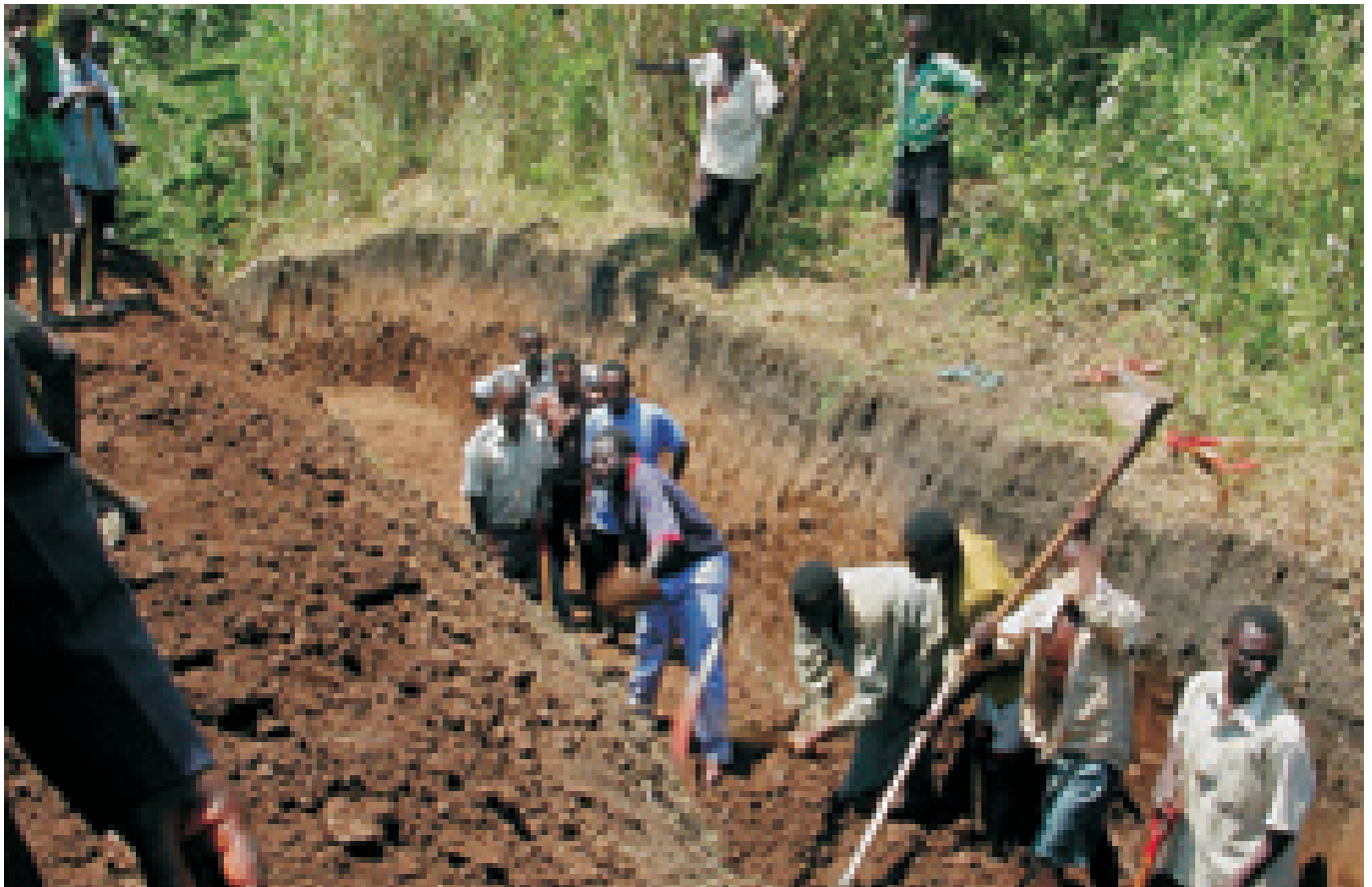
Community people help to build an elephant trench outside Kibale National Park, Uganda. The Park has entered into a number of formal agreements with surrounding communities, which allow people access to selected natural resources under certain conditions. In return, the communities monitor and protect those resources. (Courtesy Purna Chhetri)
