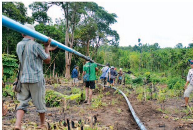
Volunteers from the village work together to bury the water pipe system
