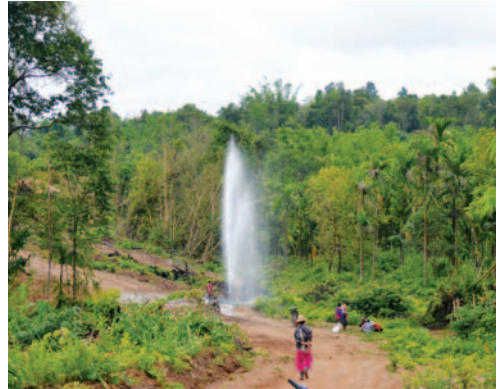
The pipe burst due to a build-up of pressure
